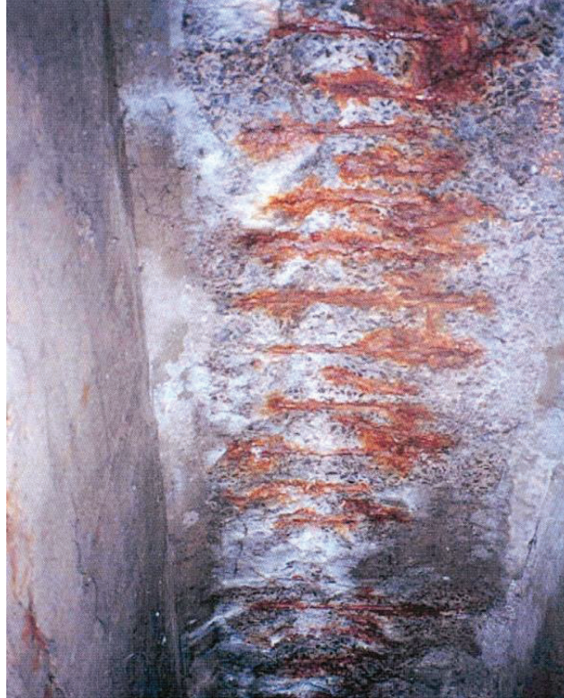
Figure 6.8 Spall and Deterioration Under the Deteriorated Concrete Slab (Monk bridge Montreal), (Zaki 2000, with permission)
