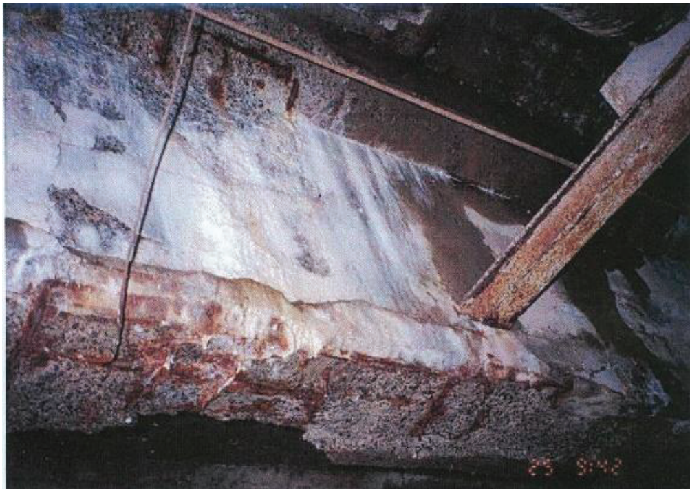
Figure 6.7 Spall and Deterioration on the Deteriorated Concrete Beam (Monk bridge Montreal), (Zaki 2000, with permission)
