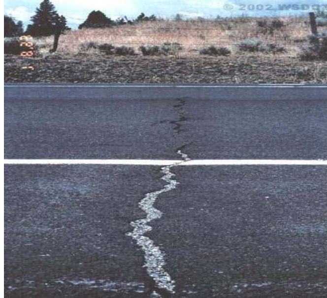
Figure 4: Transverse cracks (WAPA, 2013)
