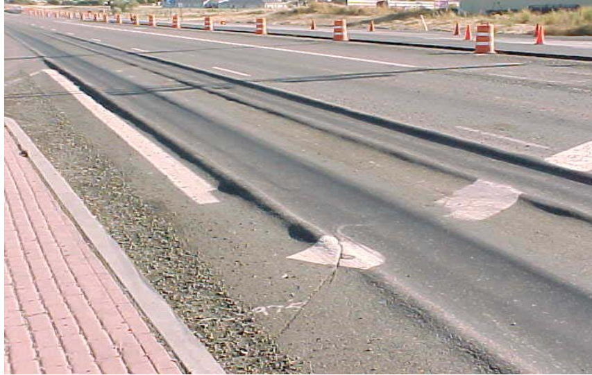
Figure 5: Pavement rutting (Pavementinteractive, 2013)
