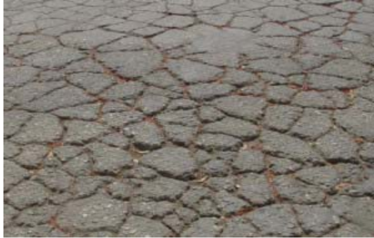
Figure 3: Fatigue cracks (Butler, 2013)
