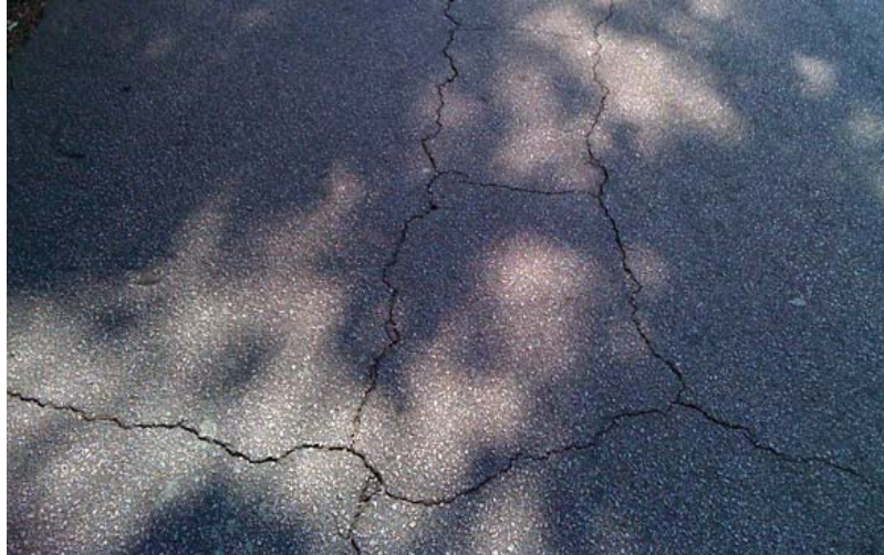
Figure 2: Block cracking (Pavemanpro.com, 2013)
