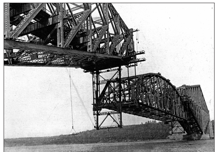
Fig. 9. The suspended truss has been jacked partly into position to complete the centre span of the Quebec Bridge. The four corners of the truss (at the base chords in tension) are connected by forged pins into vertical tension eyebar hangers that are in turn pinned into the ends of the upper tension chords of the cantilever. The temporary frames hanging down at each end were to prevent swaying from the wind.
