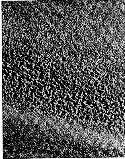
Fig. 4.1: Pitting of a steel surface [70]
