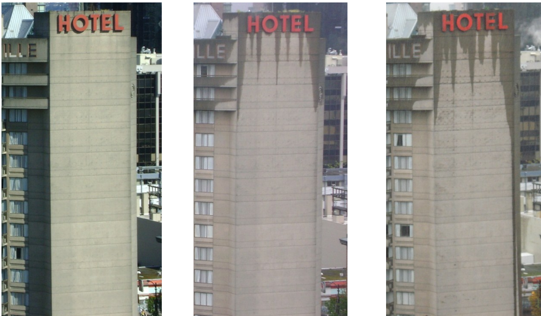
Figure 27: Sequence of photographs showing the characteristic wetting pattern of a wall of a high rise building in Vancouver with south-east exposure
