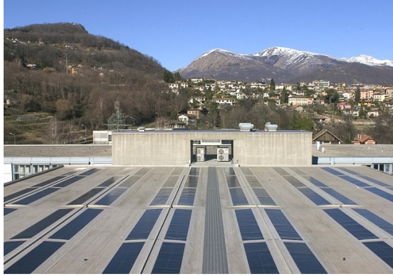
Figure 2.19. Roof BIPV systems. (a) Illustration of the installed BIPV system including (1) thin film PV; (2) white PVC membrane; (3) roof board; (4) rigid insulation; (5) electrical wire conduit; (6) the existing roof (Ban-Weiss et al., 2013); (b) Photo of a BIPV installation of thin film PV modules laminated with polyolefin membranes (Pola et al., 2007).
