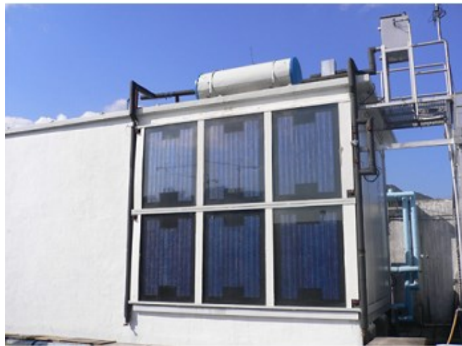
Figure 2.18. A BIPV/T water system integrated with the façade of a environmental chamber (Chow et al., 2007b)
