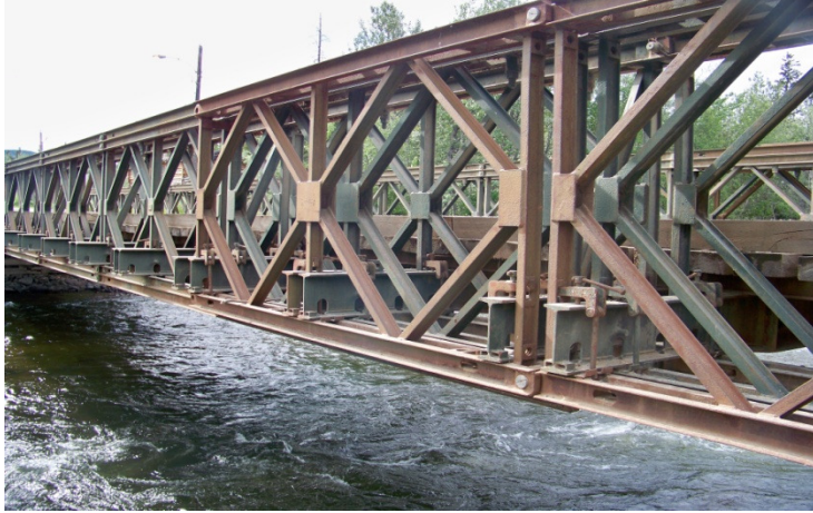
Fig. 3-9a Bridge #1 – Side View of Single-Lane Bailey
