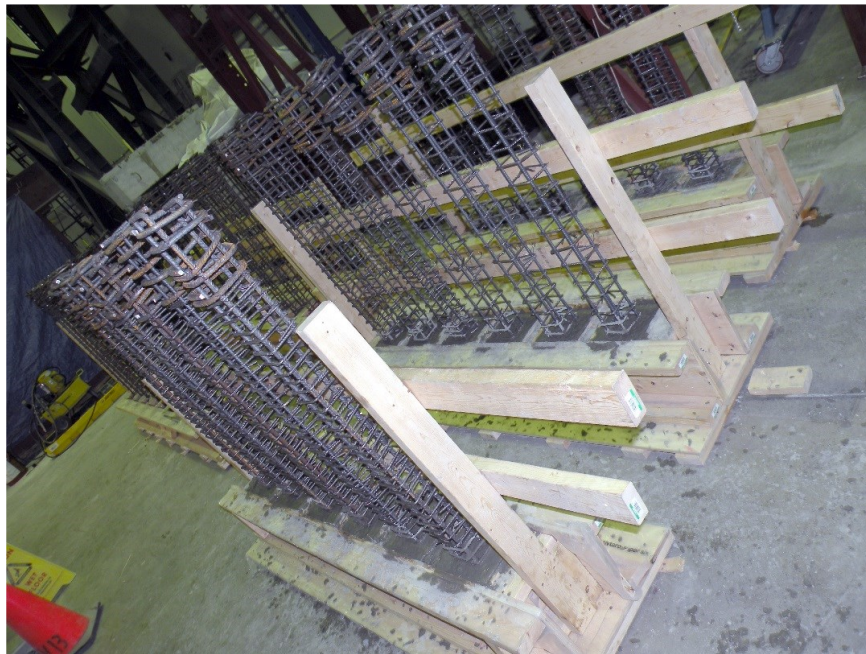
Figure A.10 Pouring the RC footing of the RMBE specimens in the timber
