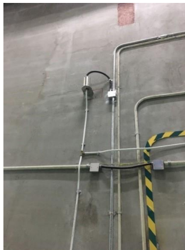
Figure 2-13: Hydrostatic levelling system used in a MUT
