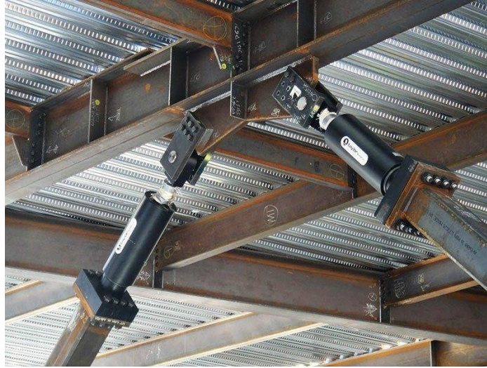
Figure 2-7 Viscous Fluid damper Installation. Source: https://www.engineering-society.com/2018/03/fluid-viscous-dampers-and-structural.html
