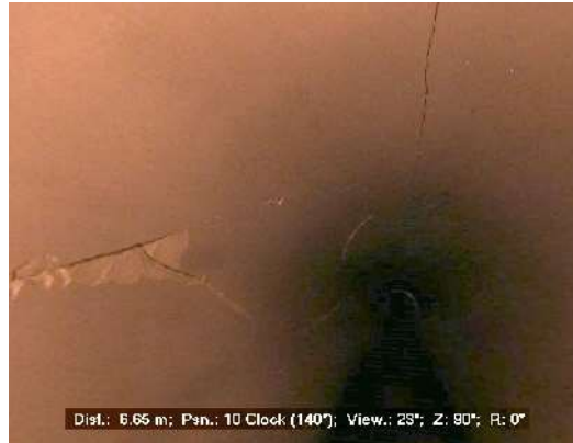
Figure 2-6. Break in sewer pipe
