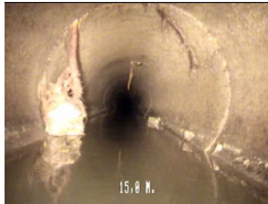
Figure 2-9. Root intrusion in sewer pipe
