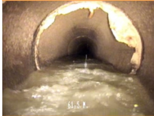
Figure 2-10. Deposit in sewer pipe
