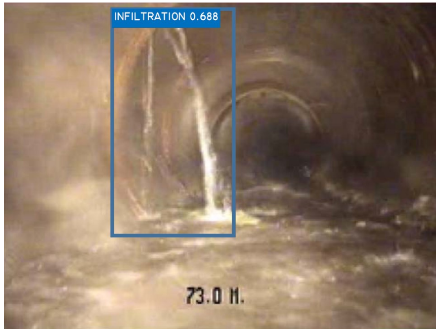
Figure 4-17. Example of image with infiltration
