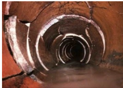
Figure 2-3. Fracture in sewer pipe
