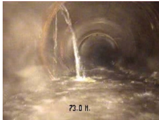
Figure 2-8. Infiltration in sewer pipe
