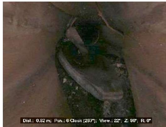
Figure 2-5. Collapse in sewer pipe
