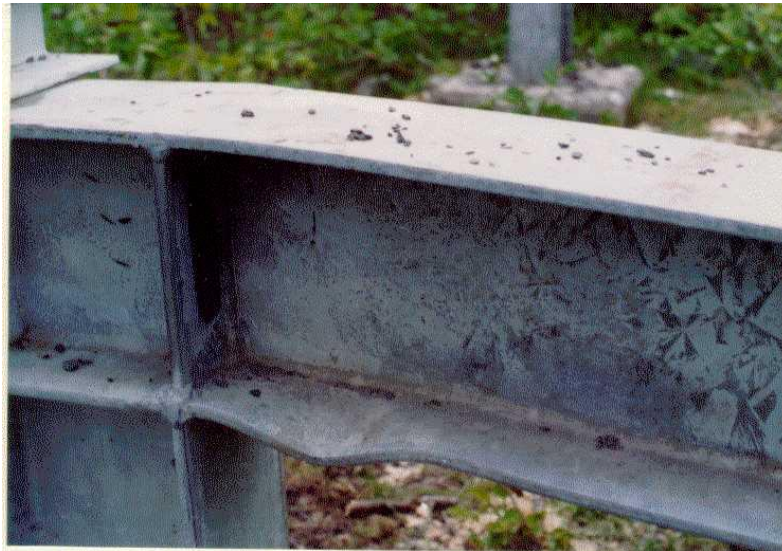
(a) Local buckling failure
