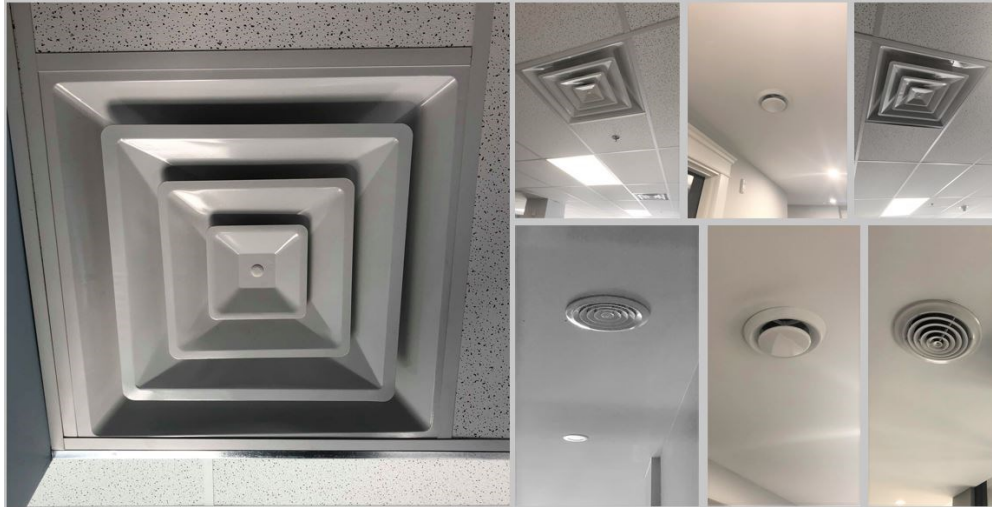
Fig. 21: Typical ceiling-mounted diffusers
