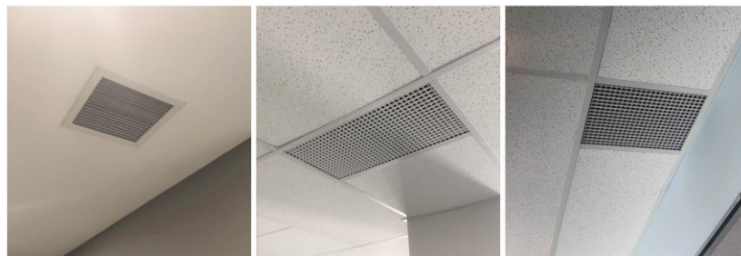
Fig. 29: Ceiling vents for mixing ventilation
