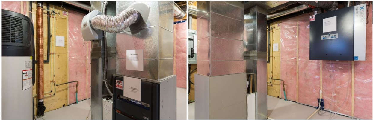
Fig. 51: Mechanical room in the basement, gas furnace and HRV (courtesy of ACQBUILT, Inc.) [59]
