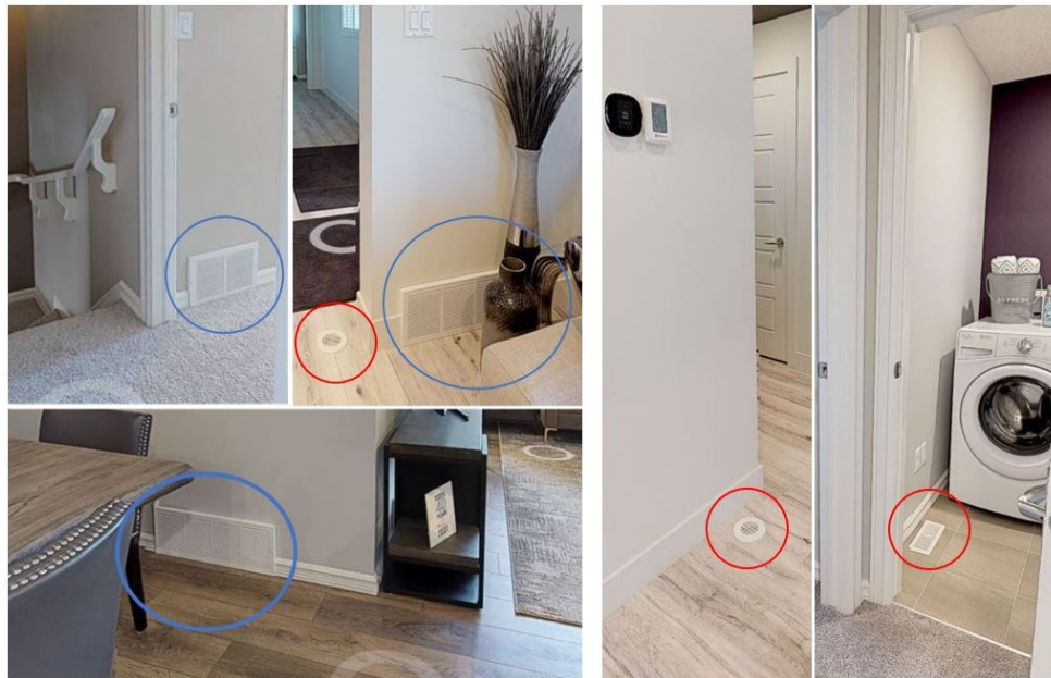
Fig. 52: Floor-mounted supply air registers and return air vents on the walls (courtesy of ACQBUILT, Inc.) [59]
