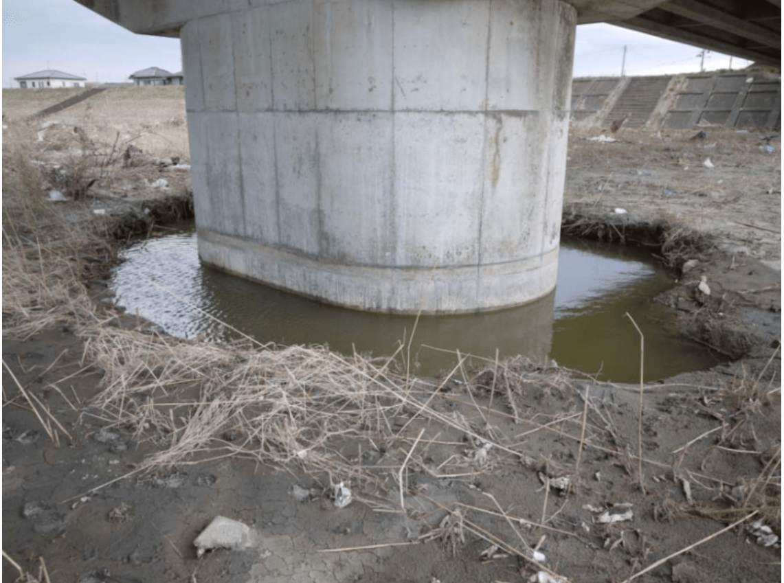
Figure 1.2: Scour hole around a bridge pier in a natural channel www.researchgate.net (n.d.)
