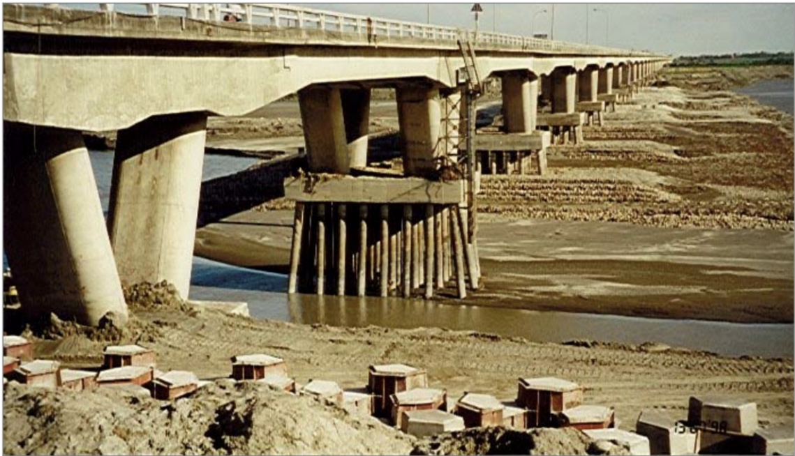
Figure 2.6: Scouring around an arrangement of cylindrical piers Pasiok and Stilger-szydlo (2010)
