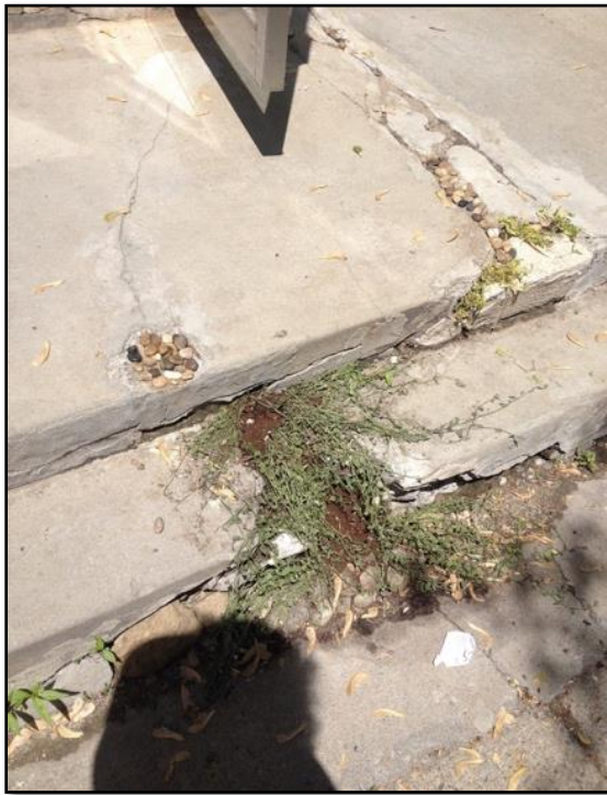
Figure 13. Front Steps at the Old Office
