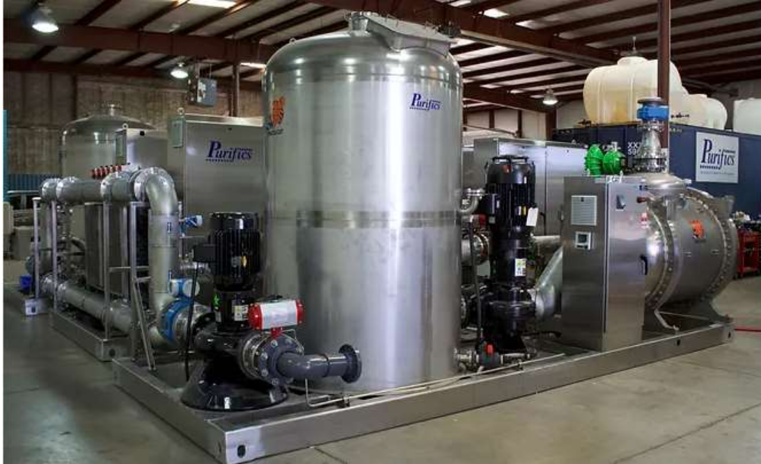
Figure 2. 12 Purifics' TiO 2 Photo-cat® reactor for water purification [111].
