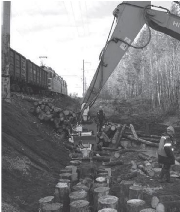
Figure 2.11. The technology of wooden pile driving in railway embankments on Peat (Zaytsev 2014)
