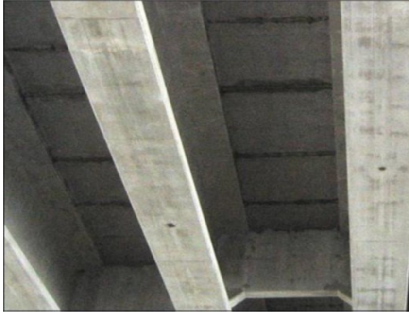
Figure 2.8 Underside of Route 123 Bridge Deck Showing Cracking (Sharp & Moruza, 2009)
