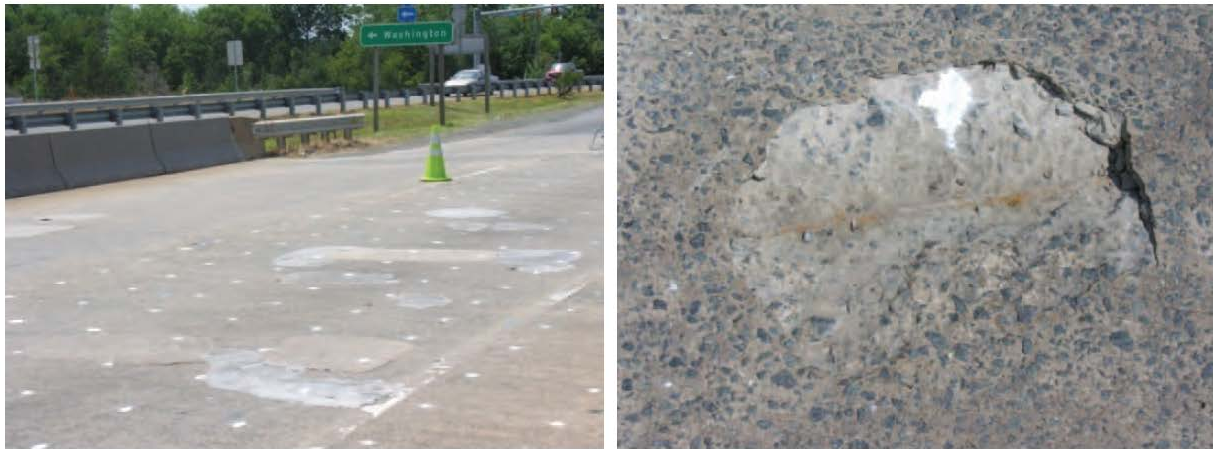
Figure 2.3 Deck deterioration (Gucunski & National Research Council, 2013)
