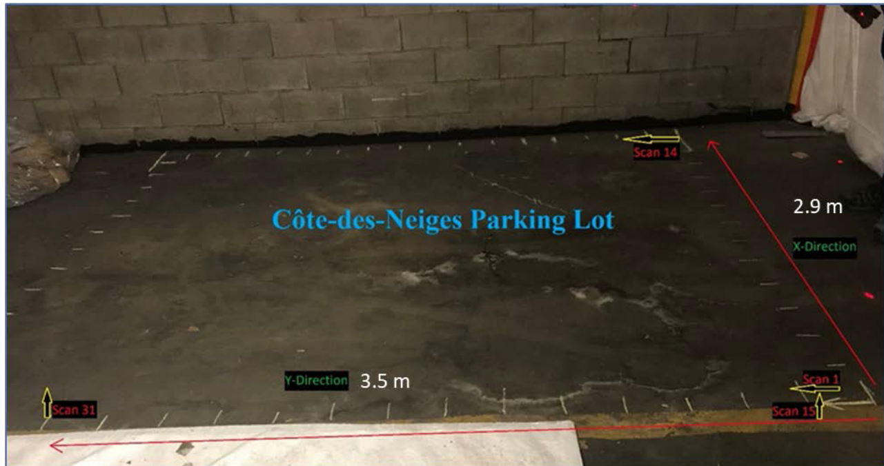
Figure 4.7 Parking lot scanned using GPR across both directions of the slab surface (Mohammed Abdul Rahman, Zayed, et al., 2022)
