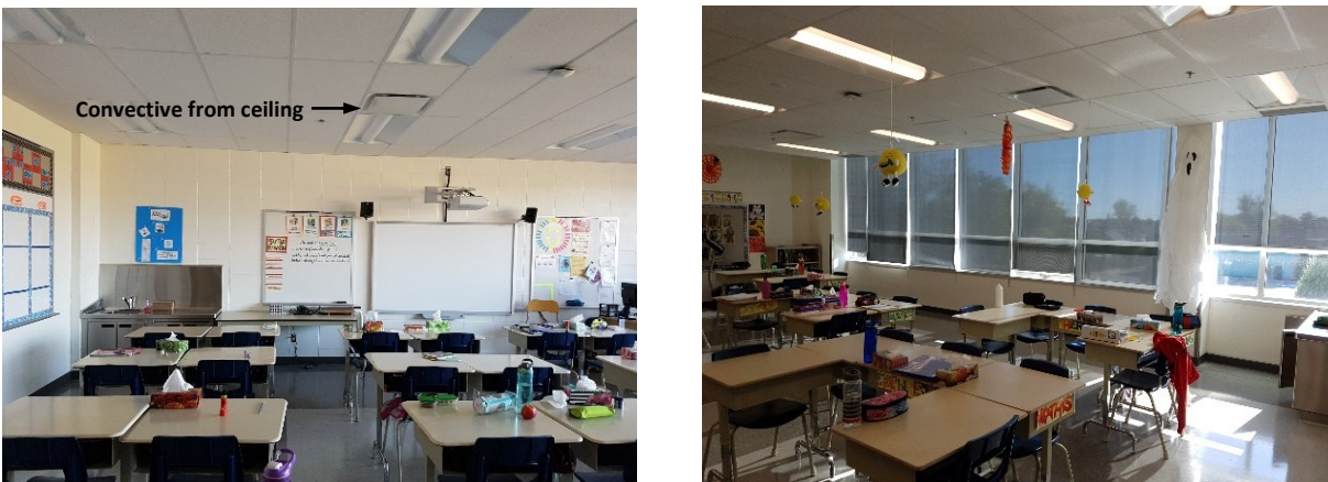
Figure 4-1: Horizon-du-Lac School – Classrooms with convective from ceiling
