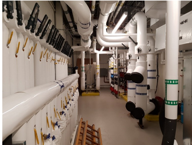
c) Mechanical room
