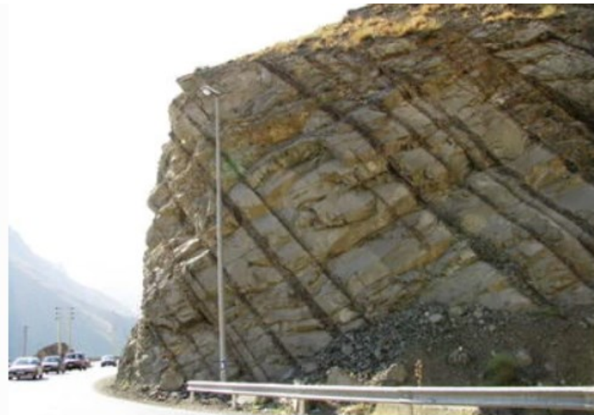
Figure 1-1: Rock slope with a potential for block-flexure toppling failure facing Chalus Road (Amini et al. 2012)
