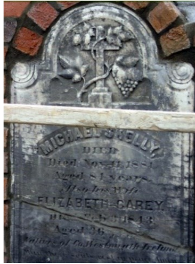
#12-Elizabeth Carey monument mounted on the wall and before cleaning. A scaffolding piece obstructs the top of the picture.
