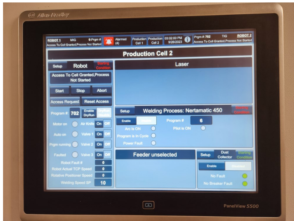
Figure 3-7 The photo of HMI screen.
