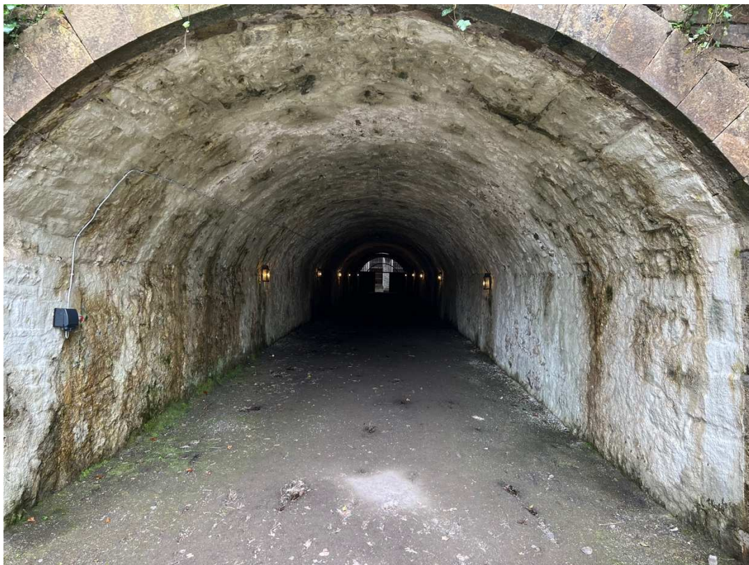
Figure 10. The tunnel leading from the area around Castle Coole’s basement to the stable courtyards, photo taken by author.
