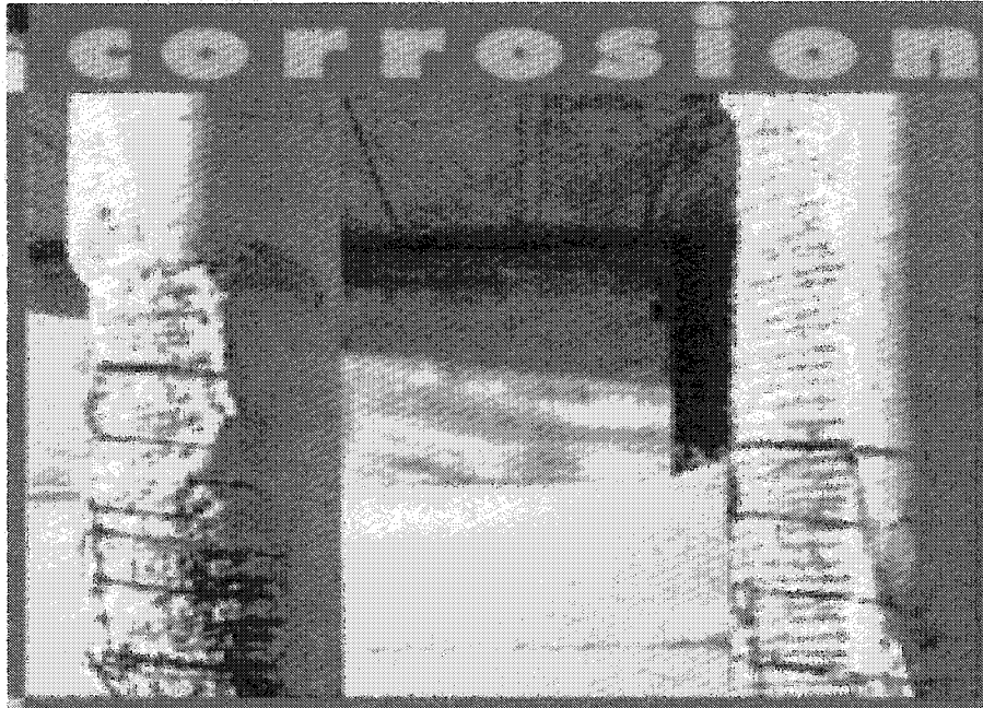
Figure 1.1 Corrosion of concrete structure
