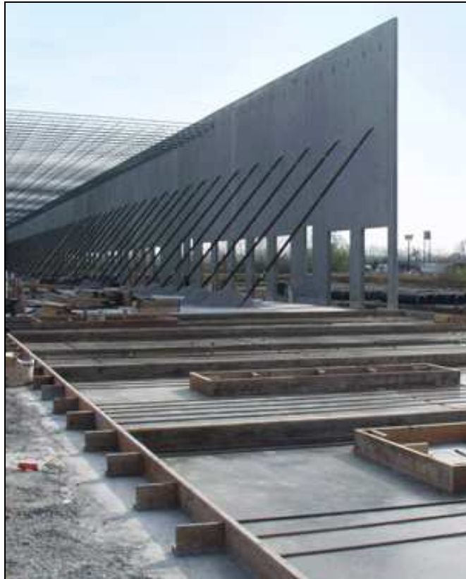
Figure 4.2 Typical Tilt-Up Panels in Building Construction (Triad Construction Company, Inc. 2009, Accessed on April 1 st , 2009: < http://www.triadconstruction.com/kansas_city_construction/news.php >)
