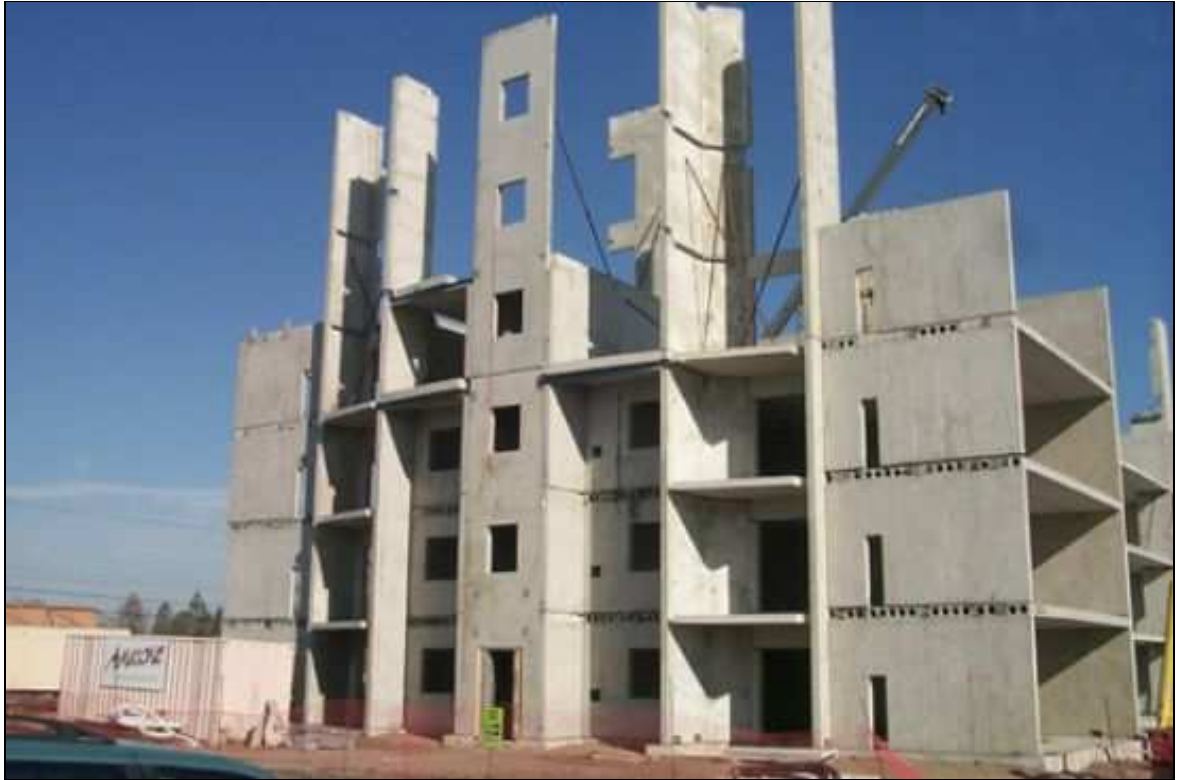
Figure 4.1 Erection of Precast Concrete Members for Residential Developments (Canadian Precasting/Prestressing Concrete Institute, Accessed on April 1st, 2009 < http://www.cpci.ca/?sc=totalprecast >)
