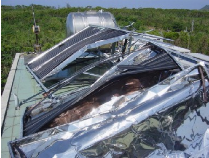
Figure 1.1.1 Damaged solar collectors (after Chung et al, 2008)
