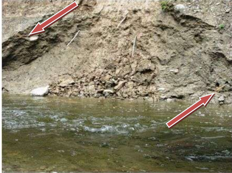
Figure 4.9 Erosion pins after one or more bank failures. Note the orange pins to the left and right of the 3 mangled pins in the center of the photograph. This photo is of a lower section of the bank in Figure 4.2.
