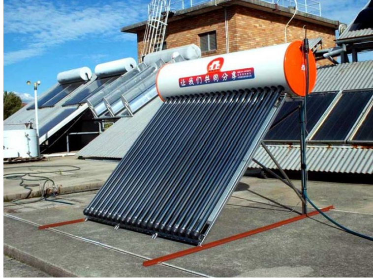
Figure 1.5: Evacuated tube solar water heater at the roof of a building of the University of South Wales (Morrison, et al., 2005)
