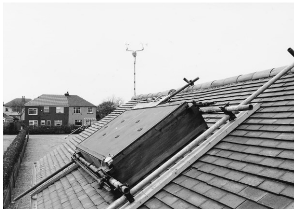
Figure 3.11: Heat transfer equipment in position on roof (Sharples & Charlesworth, 1998)
