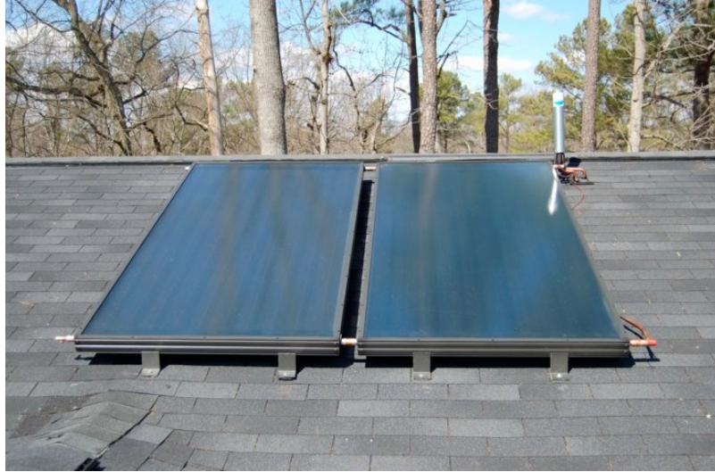
Figure 1.3: Single glazed solar-thermal collector on top of a domestic roof (Jetson Green, 2011)
