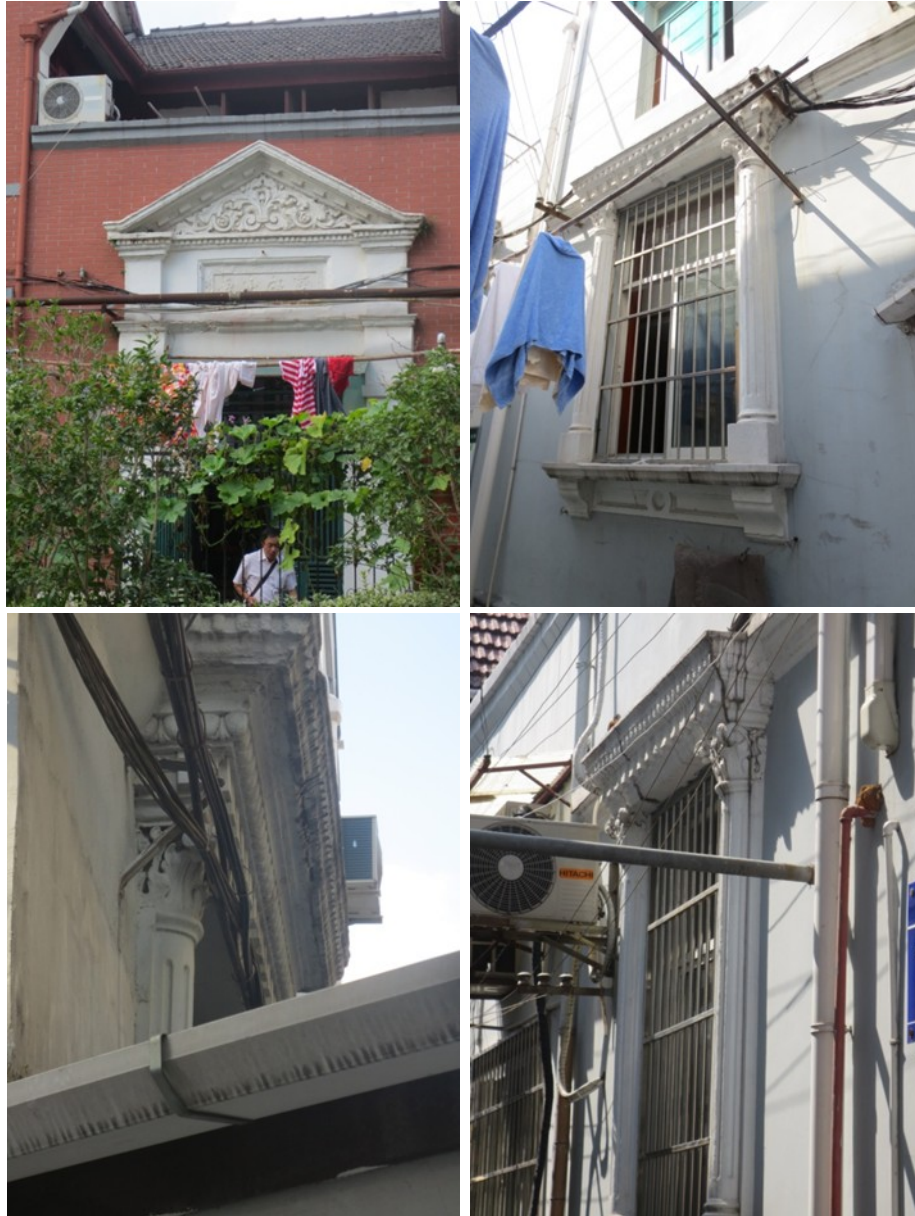
Figure 5-13: The doors and windows of New Shikumen ornamented with Western architectural elements.
