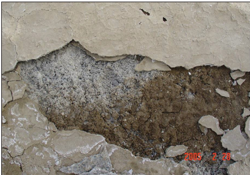
Fig. 2-15: Concrete slab of Yongan dam damaged by TSA (Mingyu et al.-2006)
