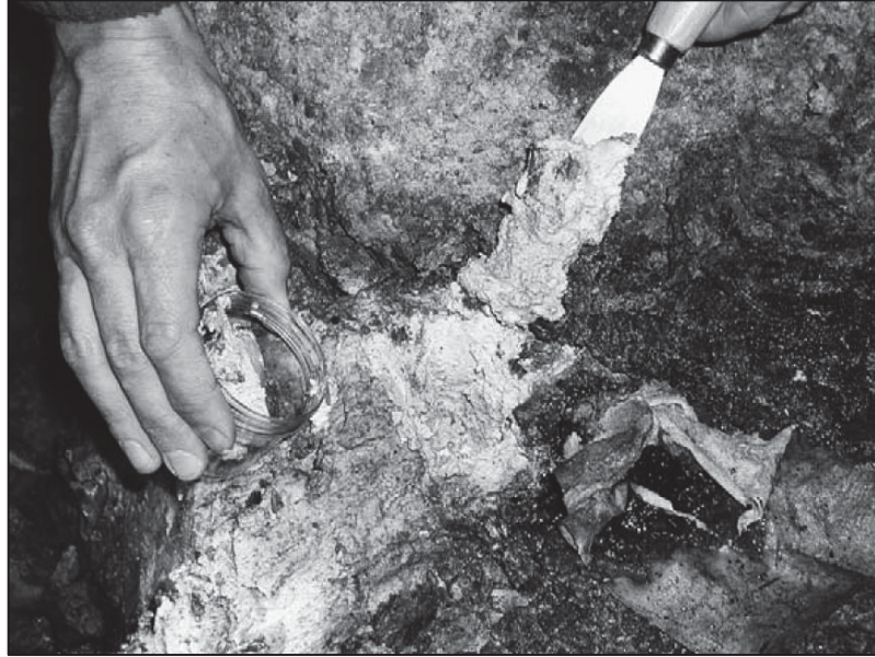
Fig. 2-13: Concrete altered into a soft mush like material on base of a tunnel lining in contact with drainage water (Romer et al.-2003)
