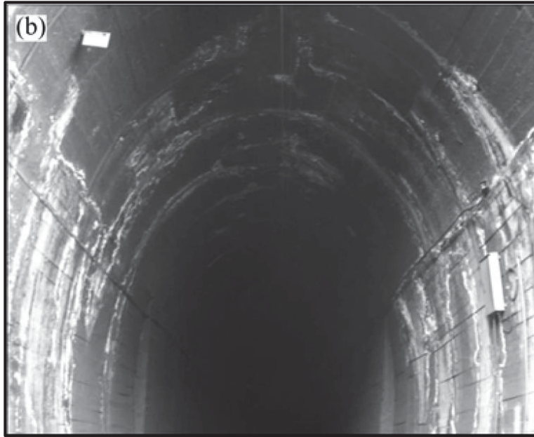
Fig. 2-16: General image of deteriorated tunnel in Chuxiong, China (Long et al.-2011)
