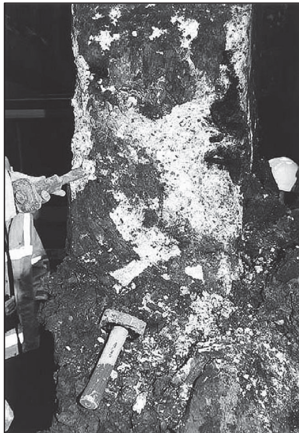
Fig. 2-8: Damage due to TSA at the base of a 30-year old bridge column (Longworth-2003)
