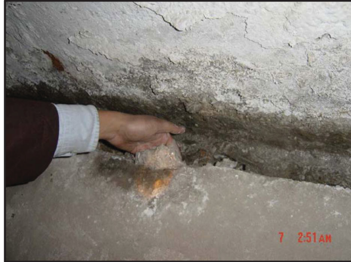
Fig. 2-14: Thaumasite sulfate attack found in drainage channels in form of development of a white pulpy mass (Ma et al.-2006)
