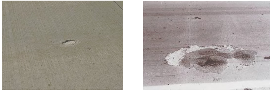
Figure 2.5: (a) Spall area < 10 square inches (left); and > 100 square inches (right) - (Project Scoping Manual, 2013)
