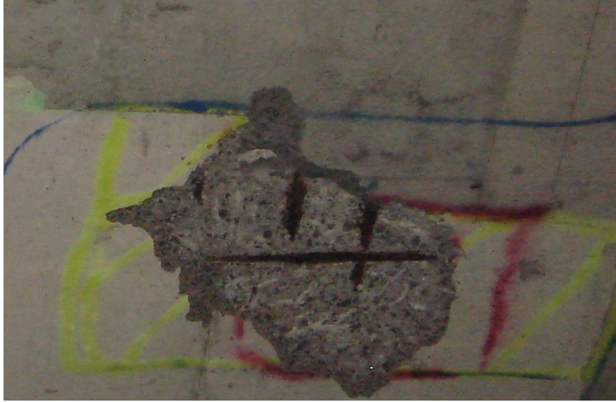
Figure: A.1 Spalled Defects in a Reinforced Concrete Structures with exposed reinforcement in a bridge in Montreal, Quebec
