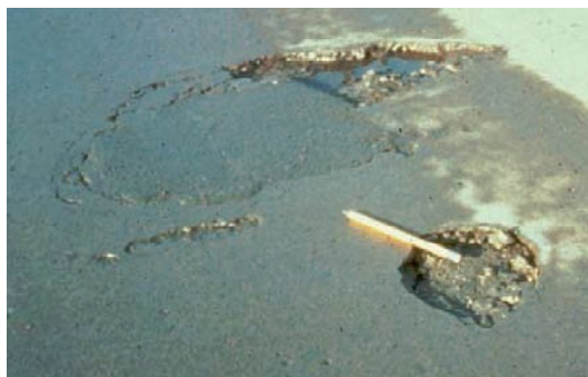
Figure 2.5: (c) Concrete deck surface scaling (FHWA 2006)
