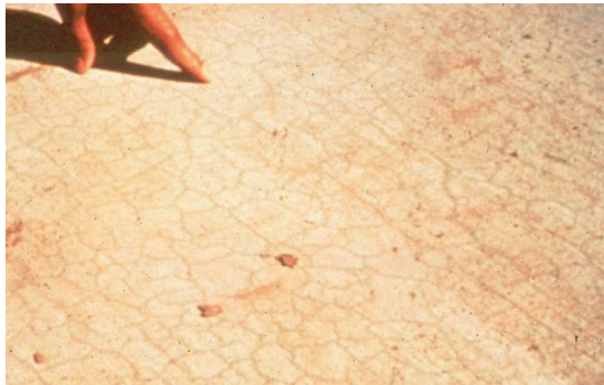
Figure 2.5: (b) Crack Map on bridge deck surface (FHWA 2006)
