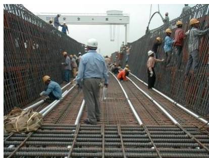
(a) Erection of reinforcement and stressing ducts of the bottom slab and the webs
