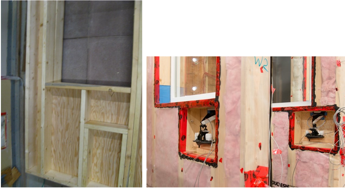
Figure 15. Left: Framing for the leakage gauge shelf of middle collection area for W2 panel. Right: Leakage gauges placed in assembled W2 and W1 panels; note the offset shelf in W1.
