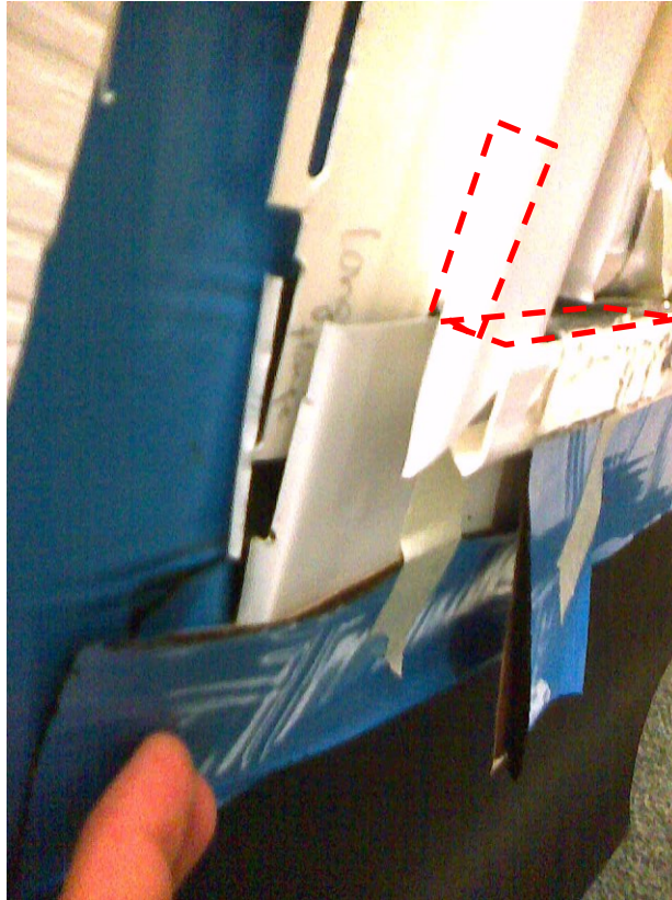
Figure 18. Sill corner collection area details for the aluminum triangular trough at W1.
