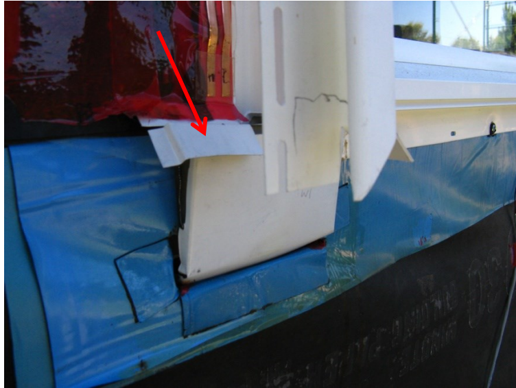
Figure 19. Additional flashing piece over the open aluminum trough at the sill corner area.
