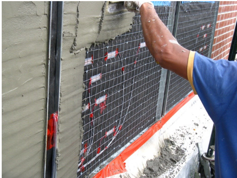
Figure 10. The application of stucco scratch coat over the metal lath on W7 panel.
