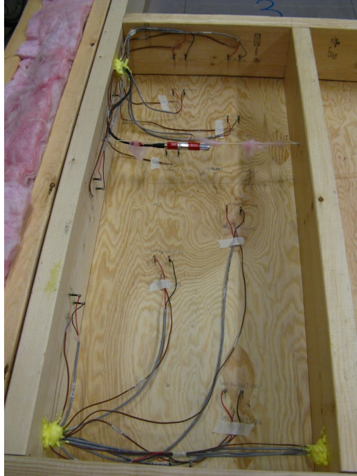
Figure 20. Typical overview of moisture pins, thermocouples, and RHT sensor installation in a wall cavity under the window sill.
