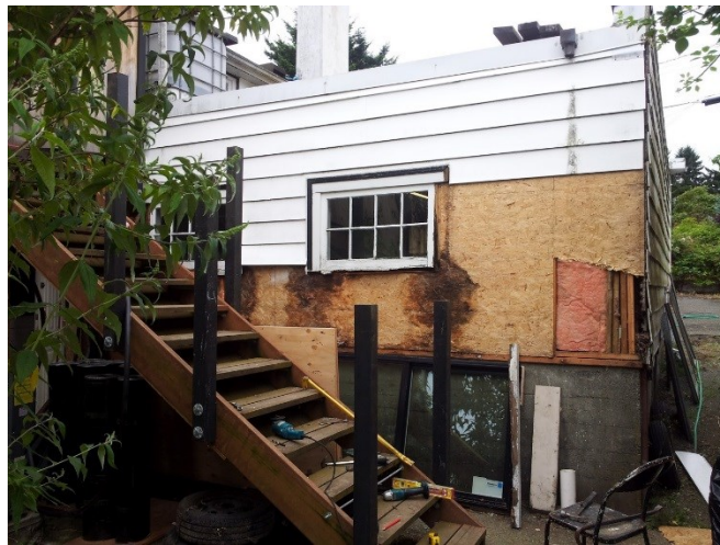
Figure 1. Sheathing board damage observed on the window sills of a wood frame wall of a garage structure in BC. Photo courtesy of David Croft (2012).
