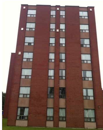
Figure 3.9 : Photo of the south-east façade of McLeod House with driving rain gauges
