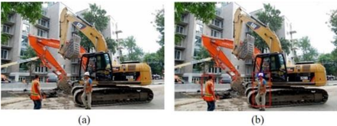
271 Figure 3-1: Identify workers without hardhats.
