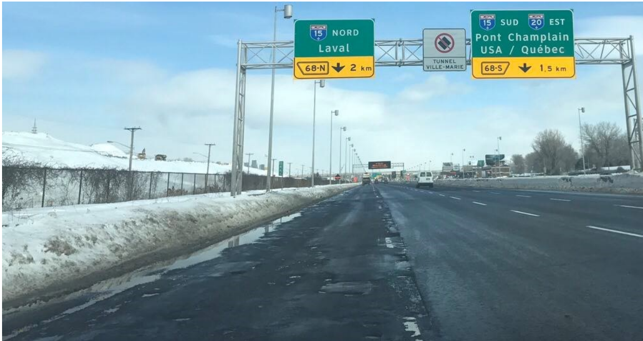
Figure 2-3 Freeze-Thaw Damage on highway 20 near exit 68
