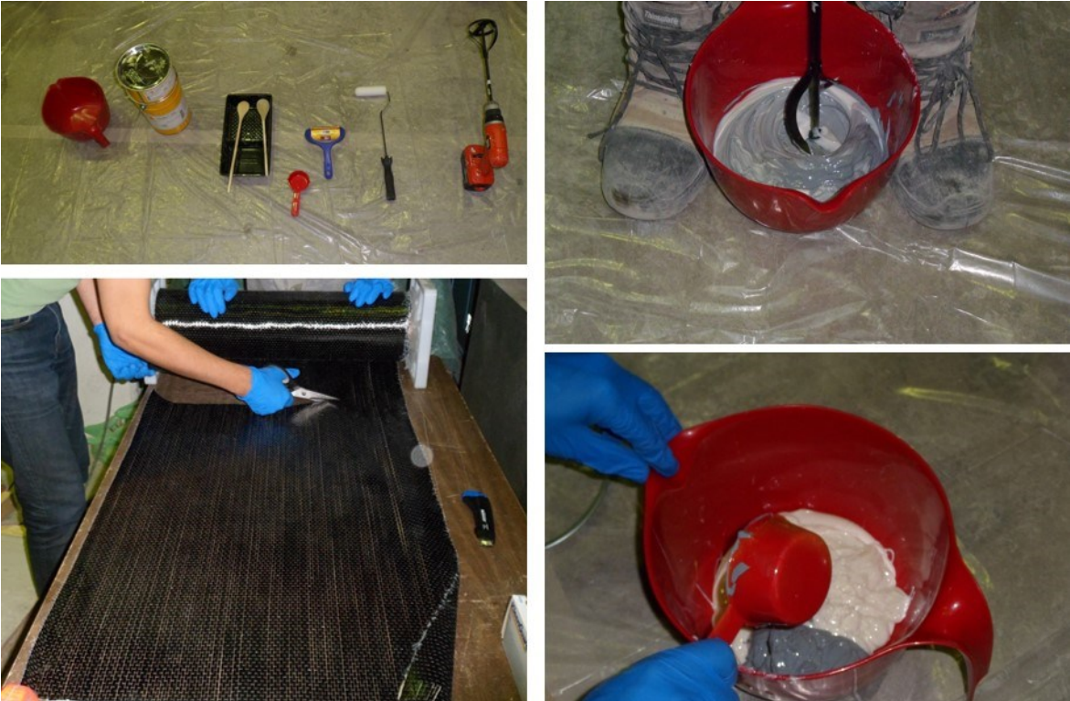
Figure A.10 CFRF sheet cutting and mixing component A to component B.
