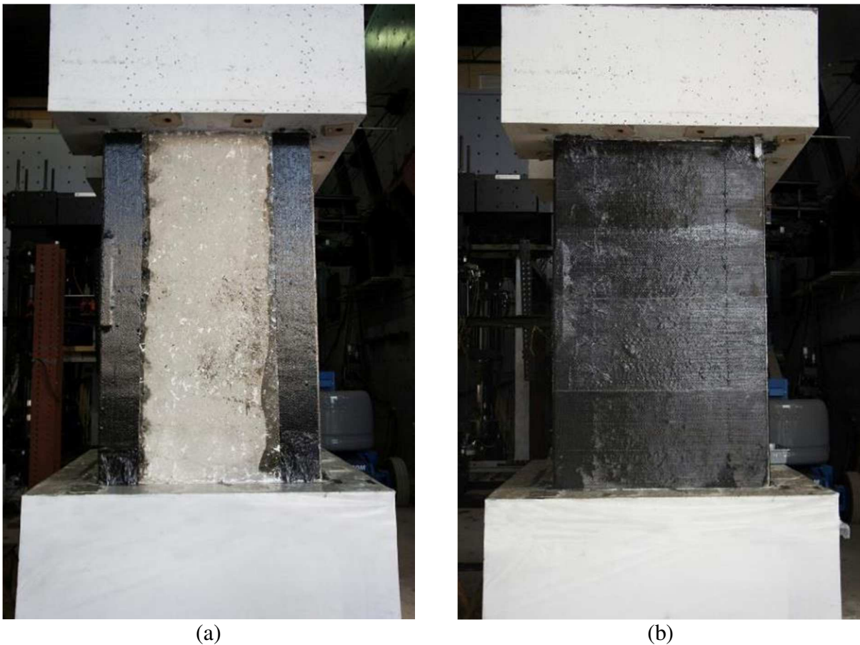
Fig. 6.16. FRP layers after installation: a) Vertical FRP strips, b) Horizontal FRP layers
