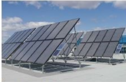
CFB Gagetown, New Brunswick, Canada 40 - G32-P Solar collectors Solar Domestic Hot Water
