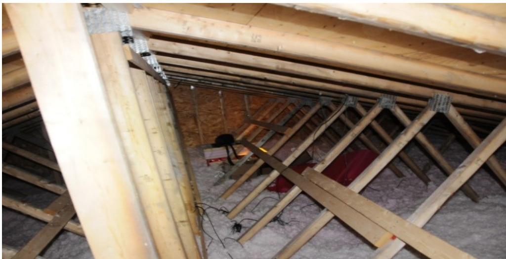
Figure 3-10. Attic view. No signs of moisture on building materials. Roofing nails not rusted.
