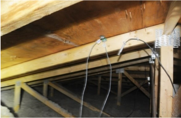
a) Sheathing wet on north slope.
