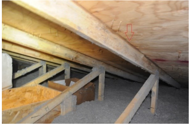
b) Moisture stains on top chord of truss.
