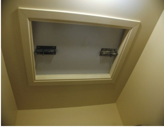
Figure 3-11. Dead bolt locks installed to ensure hatch pulled tight onto weather stripping.
