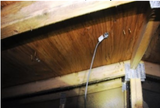
d) Sheathing wet on north slope.
