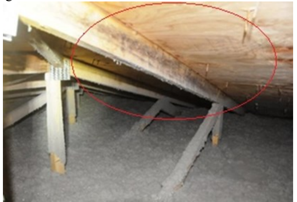
e) Black spots on truss.
