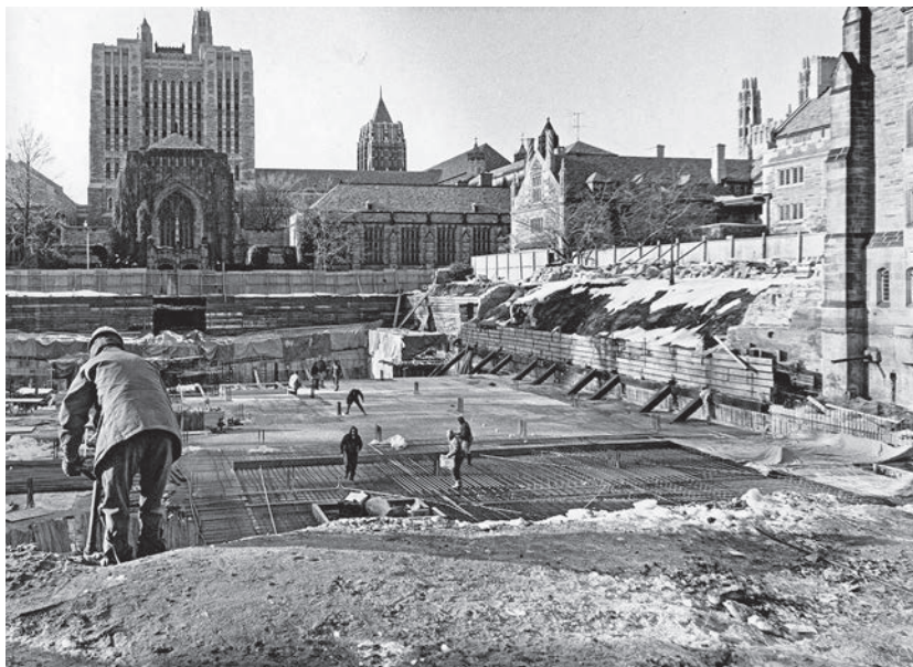
Figure 3. Cross Campus Library construction, 1968–69, with Sterling Memorial Library in the background. Manuscripts & Archives, Yale University.
