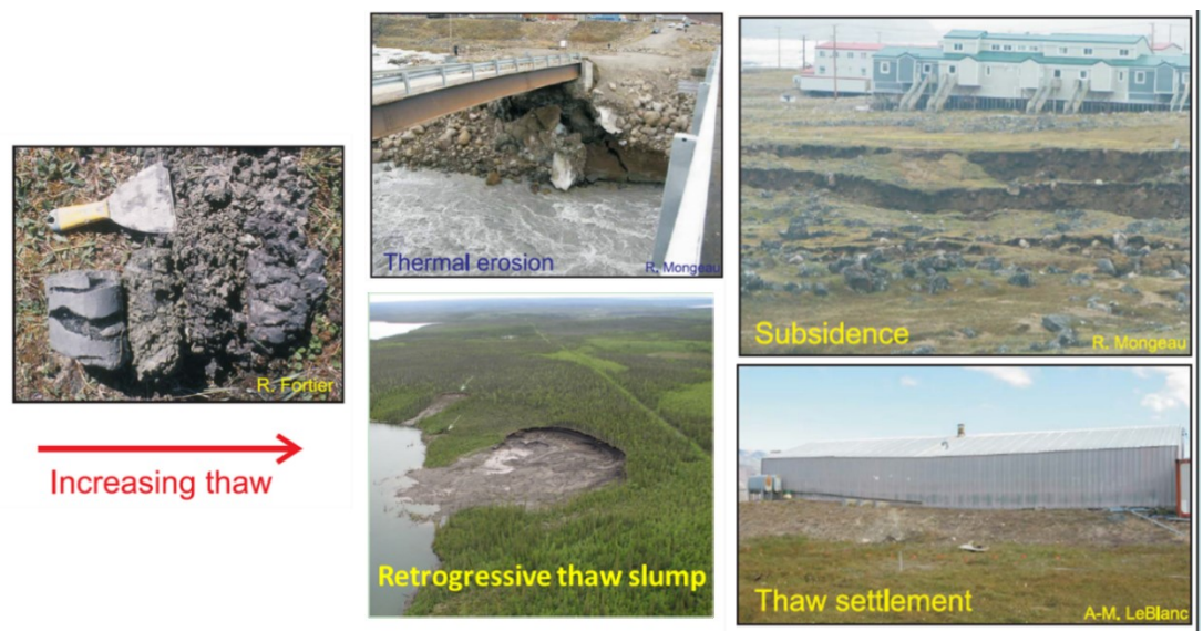
Figure 1. 2 Picture showing the impact of thawing permafrost on nature slopes and infrastructures, after Sladen (2011) and Wang (2016).
