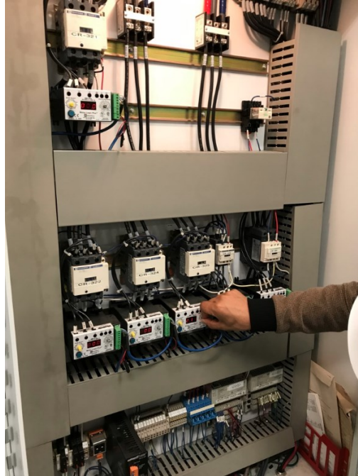
Figure 2.6: Louis-Hippolyte Lafontaine tunnel heating distribution panel.
