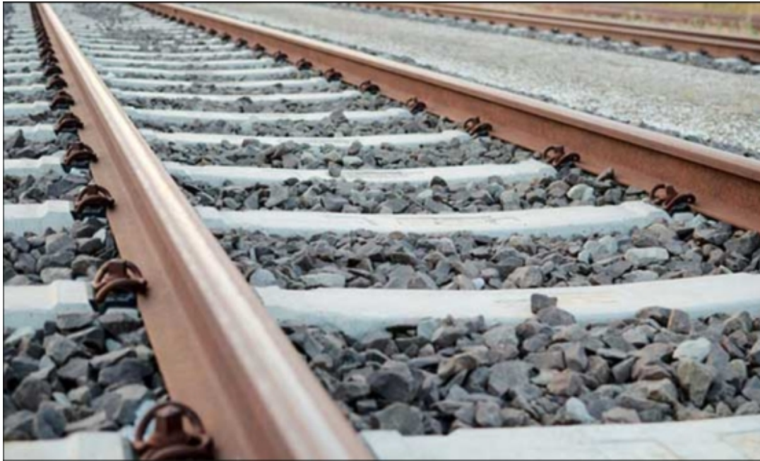
Figure 2. 11. Ballasted Track (AGICO GROUP 2020)
