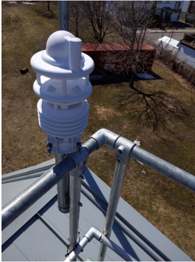
Figure 3.1.10: WS800 Weather Station secured to the guard rail at southwest corner of rooftop
