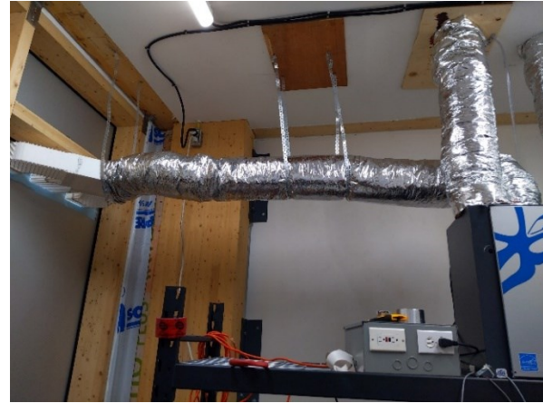
Figure 4.1.2: 3D printed manifold connected to HRV through a straight aluminum duct with flexible duct for coupling on both ends and wrapped in insulation.
