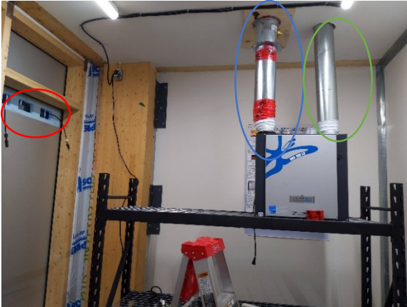
Figure 4.1.1: Opening in XPS for manifold inlet and PV connectors (red) and HRV supply air duct (green) and exhaust air duct (blue) leading to the mezzanine outside the test cell.
