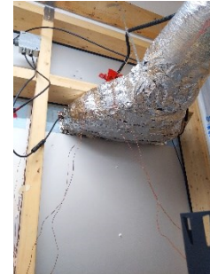
Figure 3.1.13: BIPV/T manifold insulated and thermocouples connected to data acquisition system
