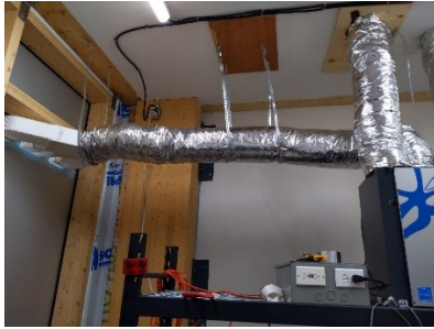
Figure 3.1.12: BIPV/T connected to the Venmar EKO 1.5 HRV through a prototype manifold and ductwork to capture the preheated cavity ventilation air
