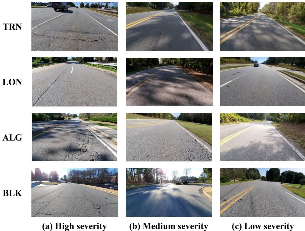
Figure 3-3 Samples of transverse, longitudinal, alligator and block cracks for three severity levels
