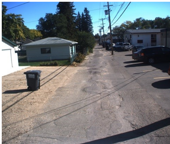
Figure 2-5 A sample image of complex defects for highly damaged asphalt pavements
