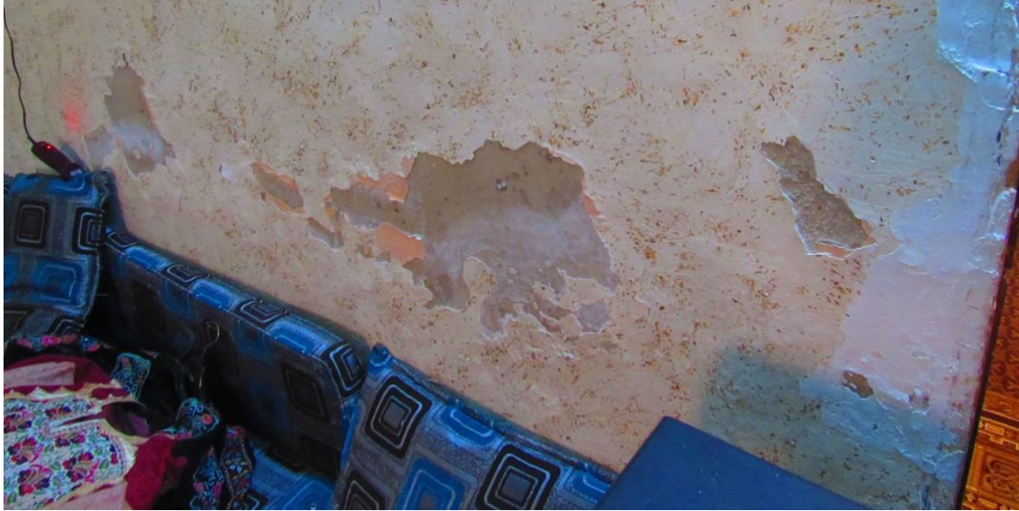
Figure 55. An example shows the effect of dampness on walls in Al-Husn camp, Irbid, Jordan (Alqub, 2022).
