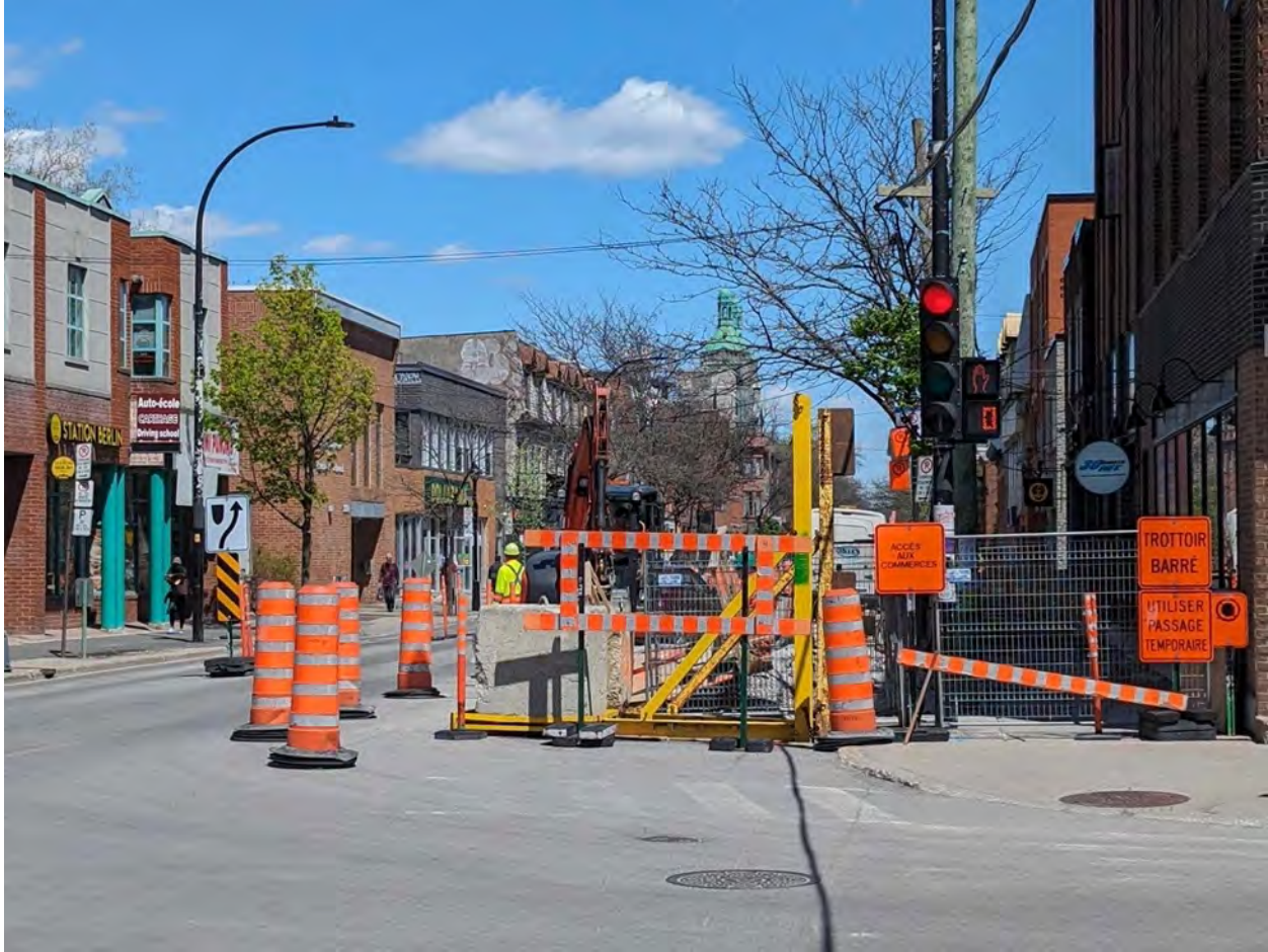
Figure 7: A typical Montréal construction blockade on Rue Centre in The Pointe. This image alludes to the ongoing changes within the built environment, and how capturing what a neighborhood is literally a moving target.
