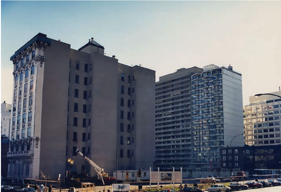
17.2 As an urban university Concordia's Sir George campus is embedded into Montreal's dynamic cityscape. A view of the McConnell Library Building being built in November 1988 shows the integrative relationship between city and university.
