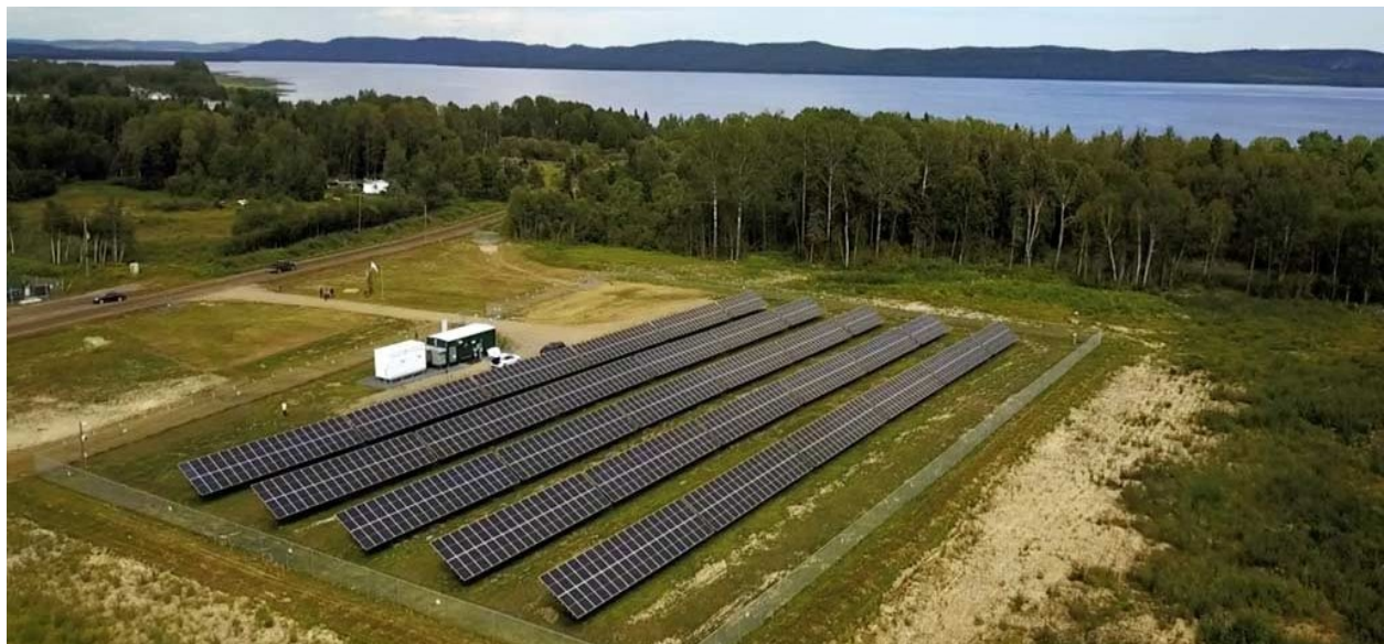
Figure 1.5 Giizis Energy Micro-grid in Gull Bay First Nation [16]
