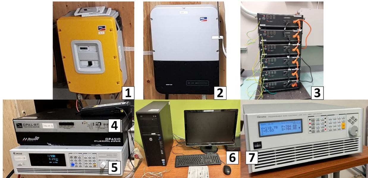
Figure 4.18 Experimental setup of the integrated system: 1) Sunny Island converter, 2) Sunny Boy inverter, 3) Battery Bank, 4) Opal-RT 4510, 5) Chroma PV simulator, 6) PC, 7) Chroma variable load.
