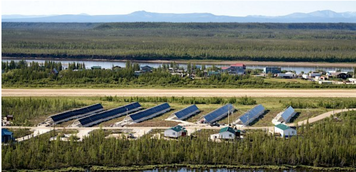
Figure 1.4 The Old Crow Solar Farm [14]
